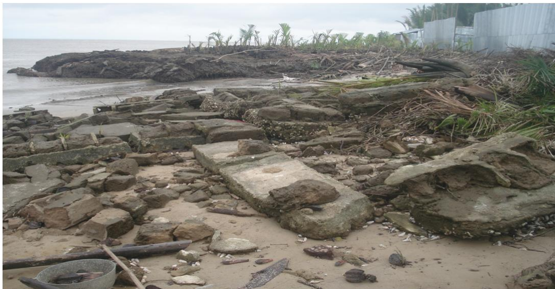
Fig. 1. Debris of brick building destroyed by sea level rise in Ibaka, Mbo LGA, Akwa Ibom state
